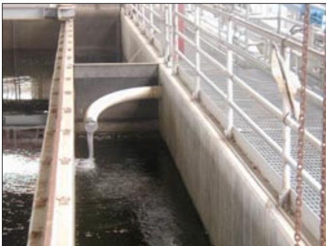
FIGURE 9.— Recovery raceway at the McNary Juvenile Fish Facility.
