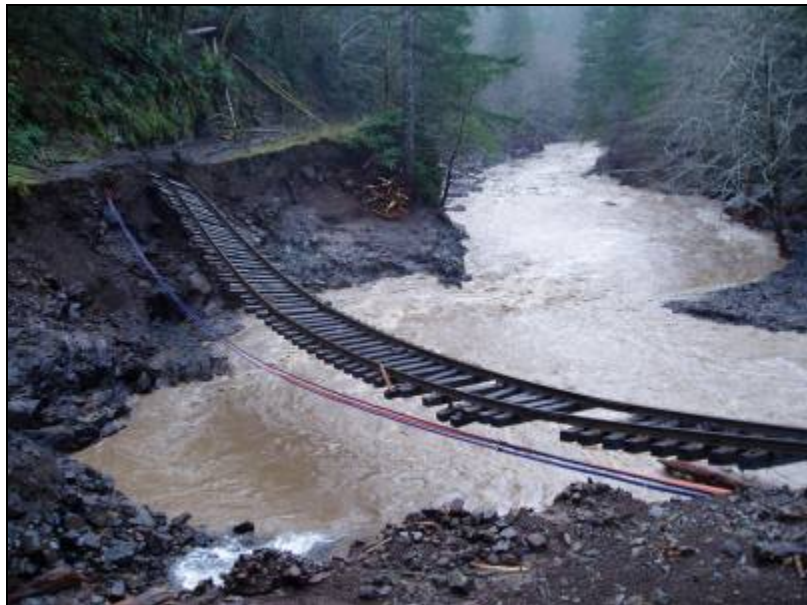
The Salmonberry River: Collapsed railroad and erosion Photo credit: Port of Tillamook Bay
