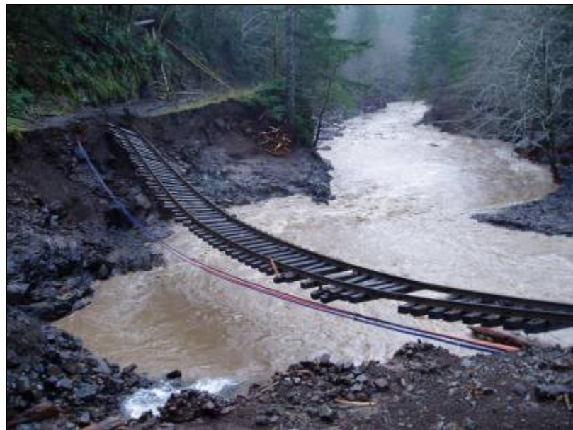
The Salmonberry River: Collapsed railroad and erosion
